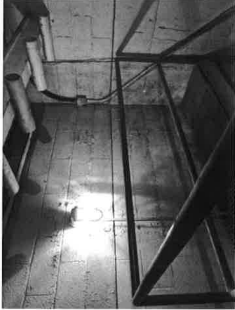
21- SEVERE HORIZONTAL CRACK AROUND ENTIRE PERIMETER
