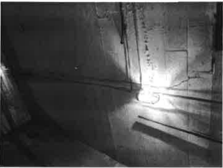
19- LARGE VERTICAL CRACK EXTENDING TO LINTEL
