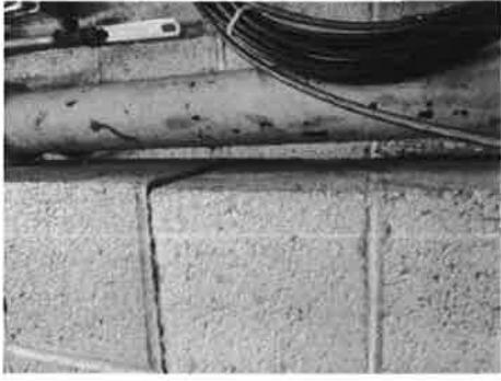
25- HORIZONTAL CRACK AT NORTHEAST CORNER OF GARAGE
