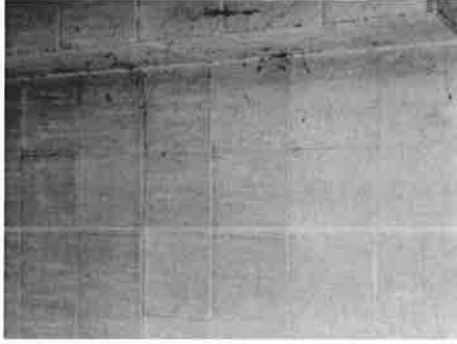
14- STAIR STEP CRACK AT CORNER
