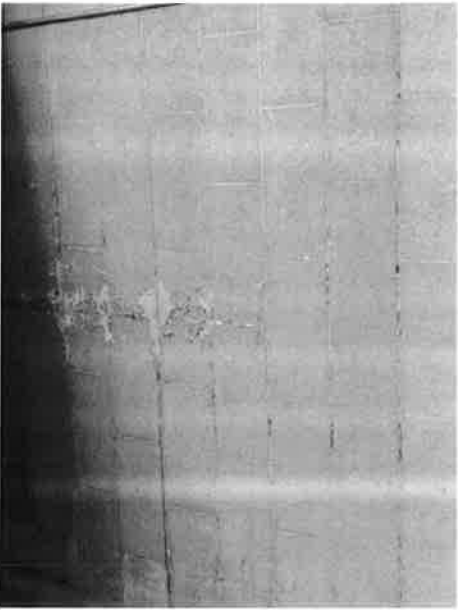
7- MOISTURE DAMAGE AND HORIZONTAL CRACKS
