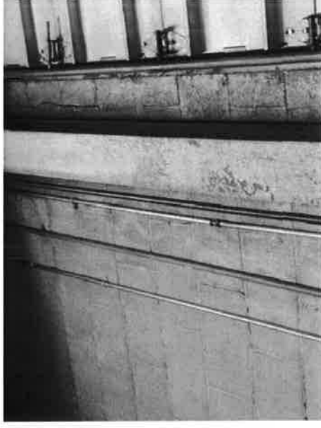
6- CRACK AT LINTEL
