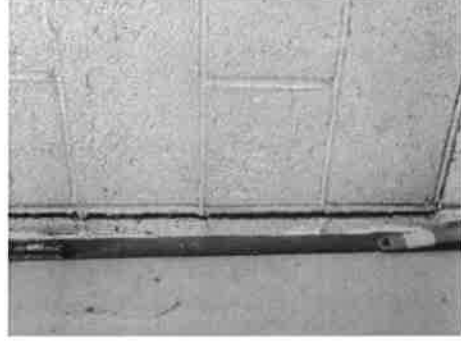
24- VERTICAL CRACK BETWEEN GARAGE AND TOWER
