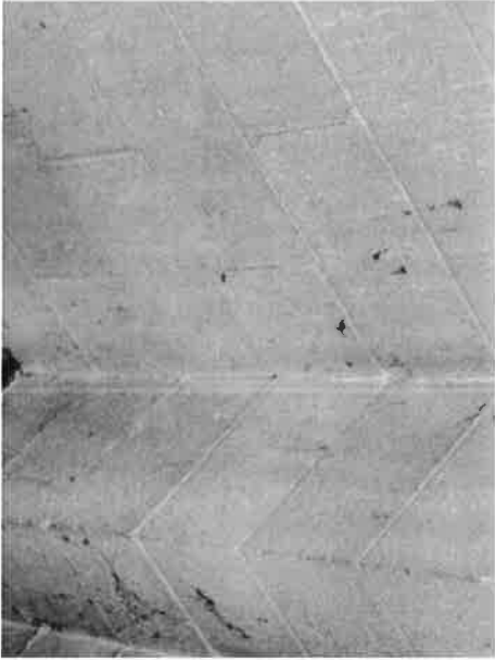
2- STAIR STEP CRACK AT CORNER
