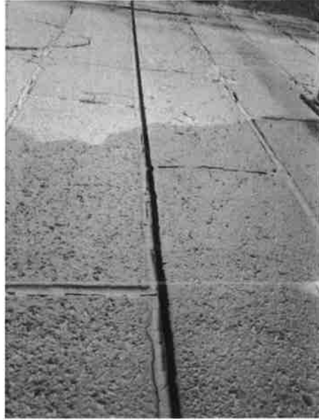
23- ANOTHER PERSPECTIVE OR HORIZ. CRACK
