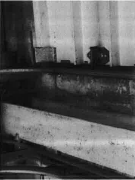
1- PIER CRACK AT LINTEL
