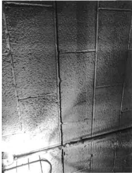
22- CLOSE UP OF CRACK
